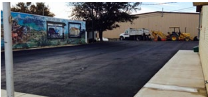
The new parking lot next to the ED building is sponsored by both the EDC, CDC and Parks Department. The parking lot has made a huge difference to the downtown area! Concrete work has been started at the Old Fields for new backstops and dugouts!
